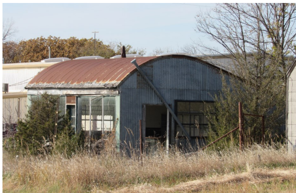
Dilapidated structures are one of the issues the Nuisance Abatement Program seeks to address.
