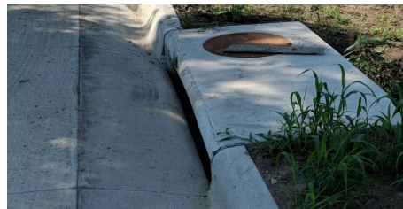
Installing or replacing 10 storm inlets were one part of Waterville’s drainage project.
