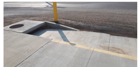
The addition of area inlets on Main Street help collect the water coming off of the road.
