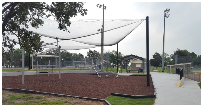
NCRPC served as the project administrator for a grant used to make improvements to the Belleville City Park.
