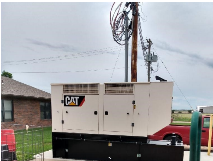
The Linn Community Nursing Home utilized the state's Community Service Tax Credits to fund a project for a new generator, HVAC and plumbing.
