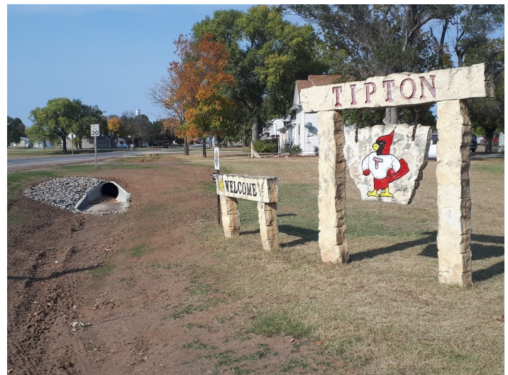
The City of Tipton completed a project in 2020 that improved the city's storm drainage system by installing new culvert pipes, a portion of enclosed storm sewer, area inlets, ditch grading and minor street repairs.
